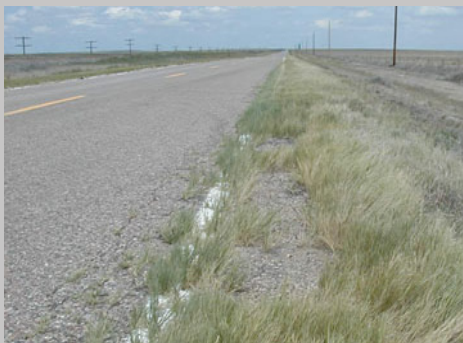
Overgrown highway shoulders
