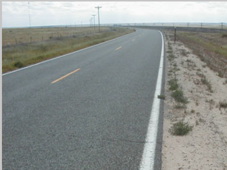
Inadequate highway shoulders
